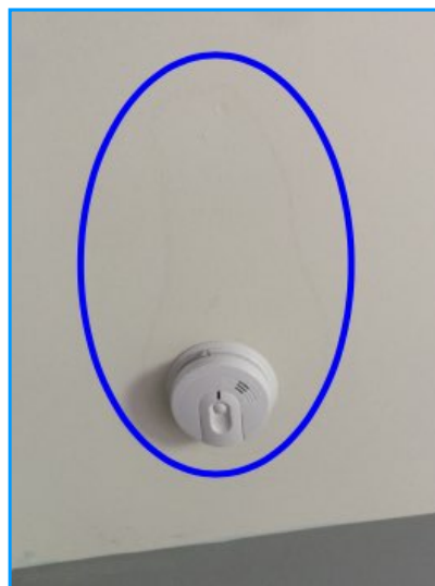
Staining on ceiling under attic air handler.
