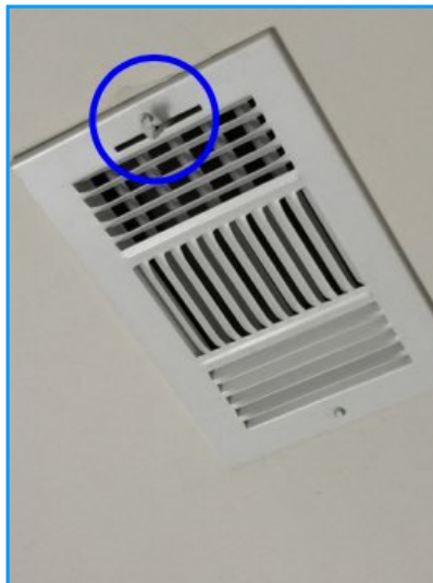
Bent adjustment lever won't allow vent to be closed.
