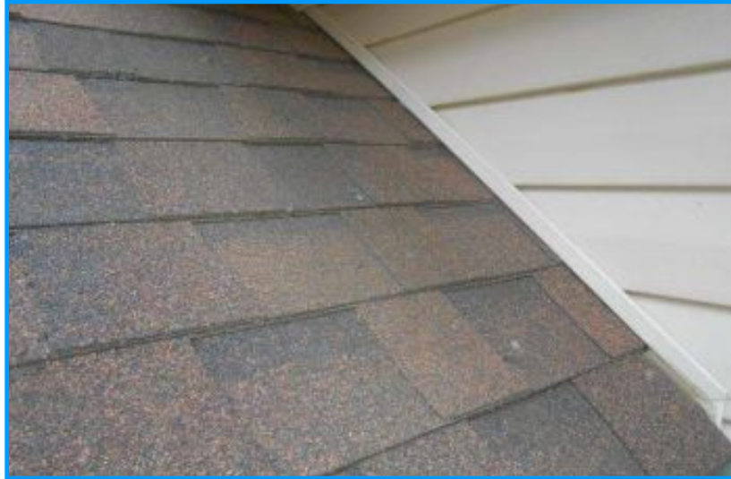
Exposed nail heads.
