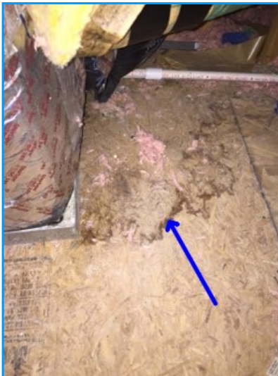
Air handler staining on sub floor
